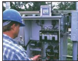
4501 Pump Station Monitor
